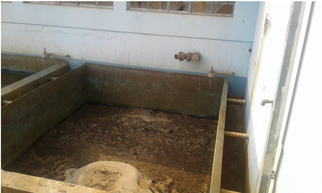
Picture 15: Sand filters needing sand replenishment
