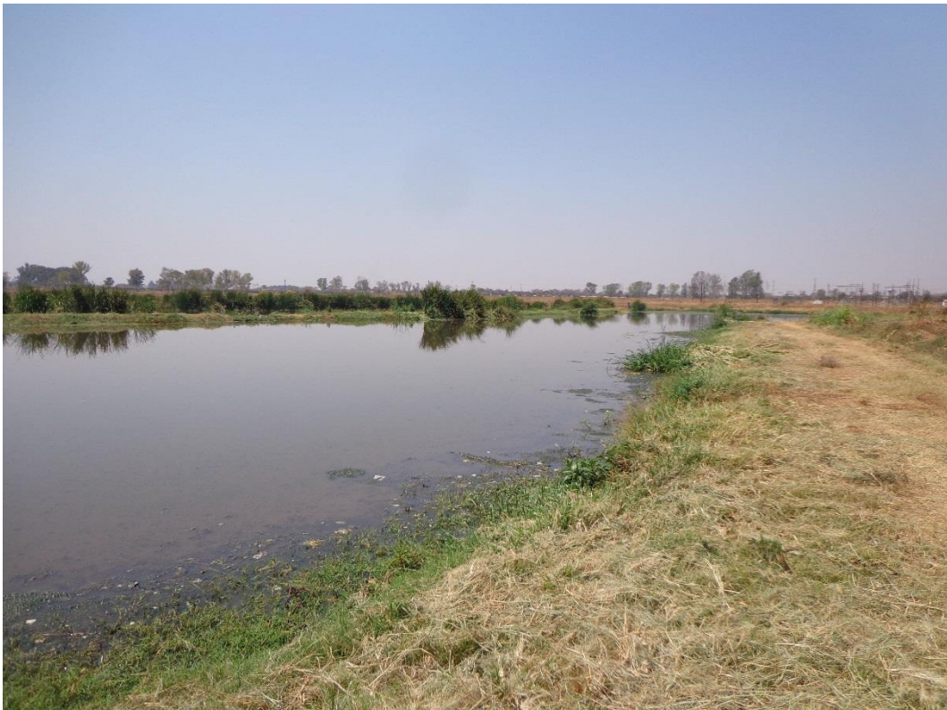
Picture 21: Sewage overflow at Kaguvi 1&2 pump station
