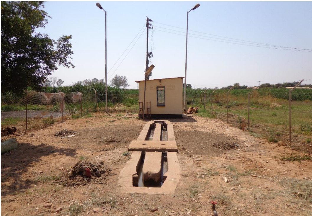
Picture 17: ZMDC pumping station
