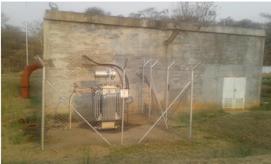
Picture 12: Clifton Pump station
