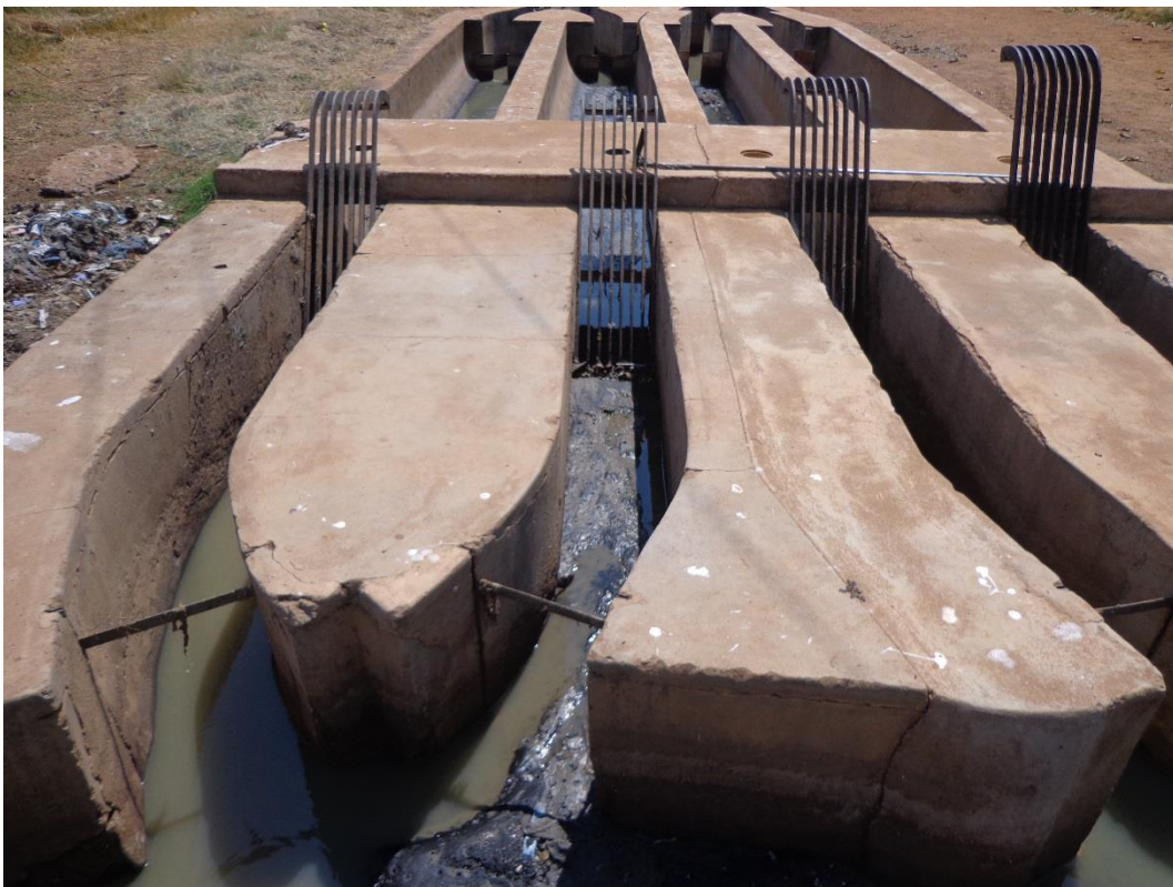
Picture 19: Grit collection at ZMDC sewage ponds grit channel.
