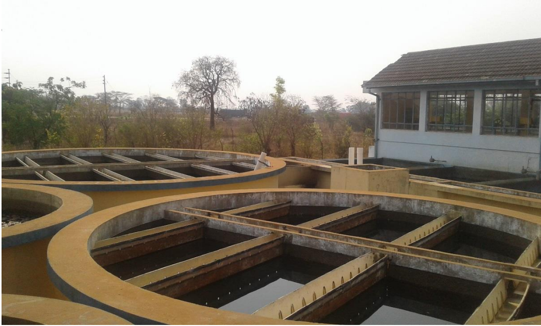
Picture 14: WTP Circular Clarifiers
